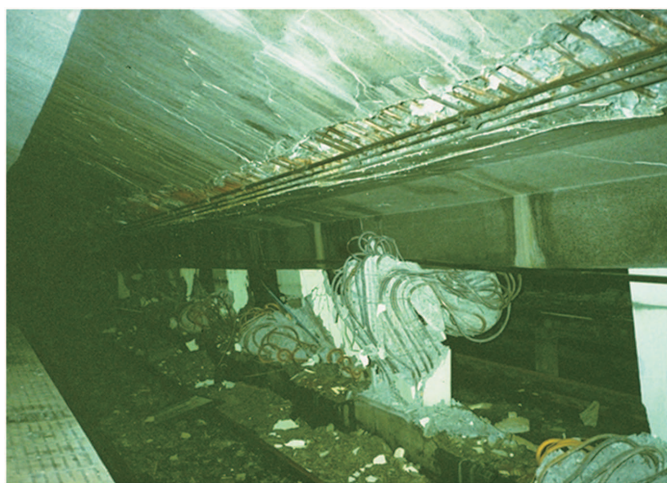
Fig. 2. (Color) Compression failure of the central columns of the Daikai Station subway structure. (Reprinted with permission from Sakurai 2014.)
