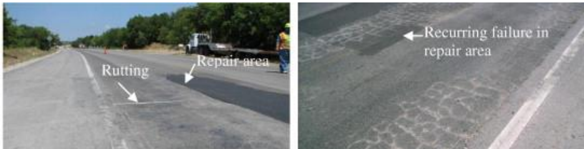
Fig. 1.3 Recurring failure in repair area (Chen et al., 2013)
