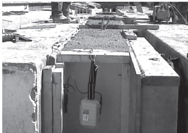
Fig. 2.2 Temperature recorder suspended from structure
