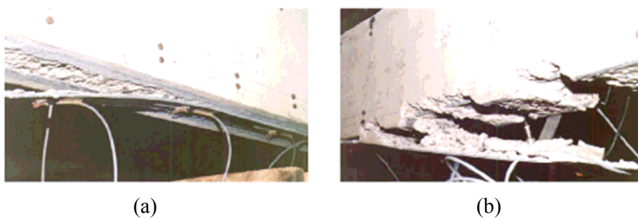
Fig. 2.4 FRP Delamination failure mode (a) without concrete cover, and (b) with concrete cover (Renata et al. 2008)
