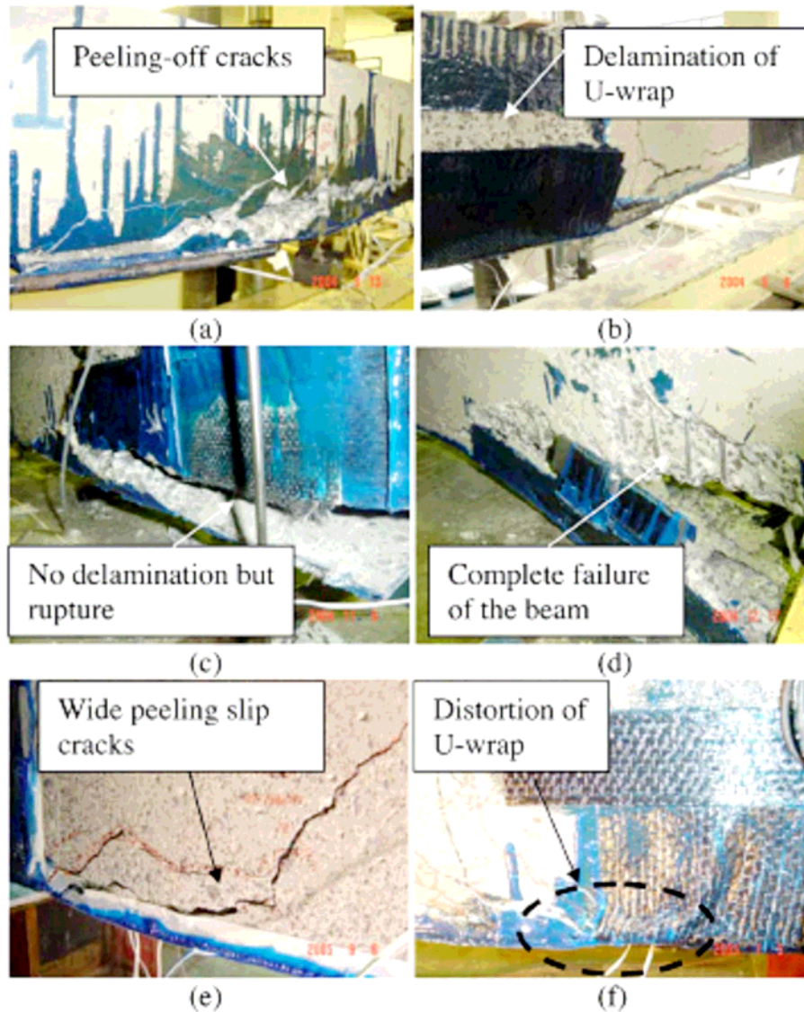
Fig.3.9 Failure modes of the beams shown in Fig.3.7: (a) J-1 with permanent metallic anchor; (b) J-2 with nonanchored U-wraps; (c) J-5 with mechanically anchored U-wraps; (d) J-6 with mechanically anchored prestressed U-wraps; (e) J-7 without side sheets; and (f) J-9 with CFRP-sheet anchor and without side sheets (Kim et al. 2008a,b).
