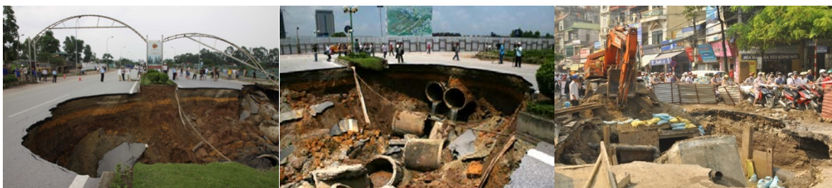
Figure 2.12 Cave-ins and road collapses in Hanoi city
