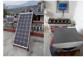
Fig. 5. Solar Backup Units in Pokhara Base
