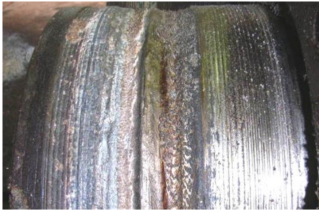
(b) Eroded surface of rotor
