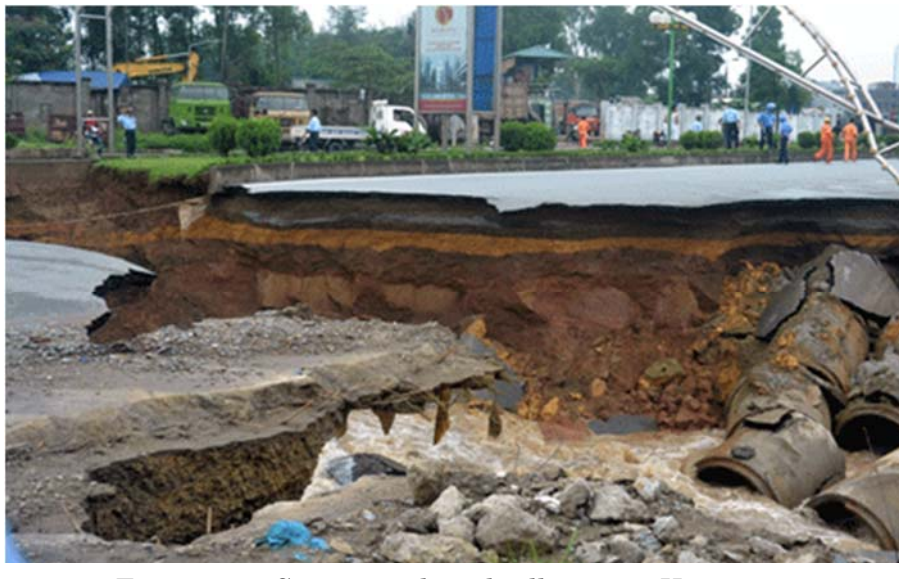
Figure 2.10 Cave-in and road collapses in Hanoi city
